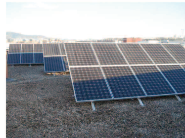
Photovoltaic solar panels
